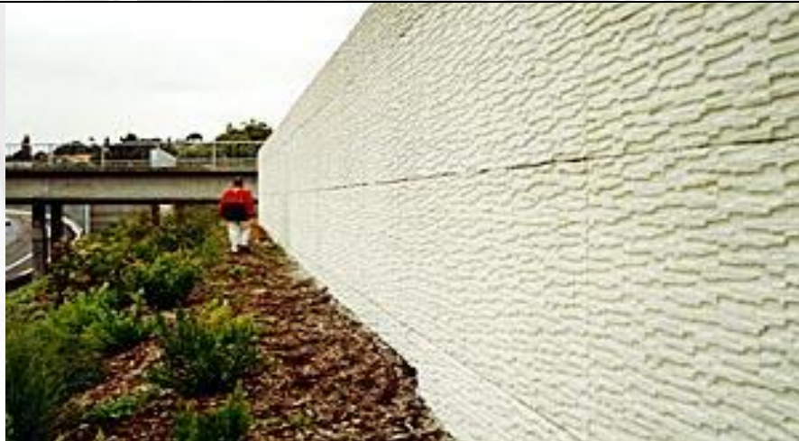
Australia, Stacked Panels, 混凝土式
